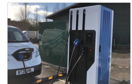
DC EV chargers
